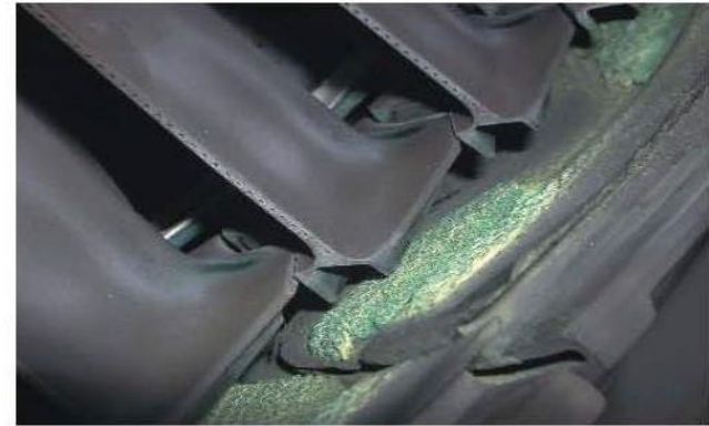
HP Seal Segments showing severe thermal erosion
