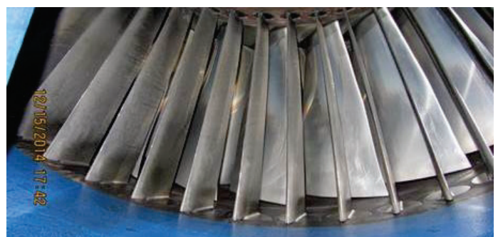
Figure 11: E12 Filtration after 6,500 Hours (No Washes)
